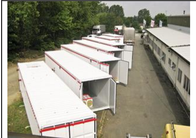
Fig. 4. Containerized treatment system with three-phase decanter getting prepared for shipment
